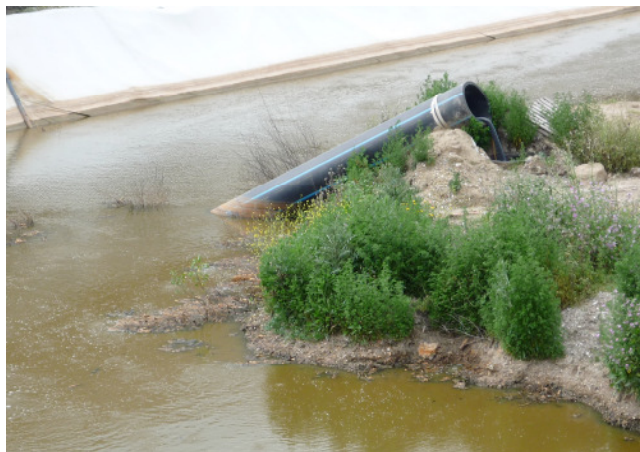
Figure 13: Buried landfill from the Uttaro dumpsite, showing obvious non-conformity (leachate and a broken chimney for gas expulsion) to safety requirements
